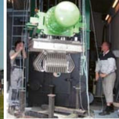
Left: Installation of a Stirling motor for combined heat and power.
